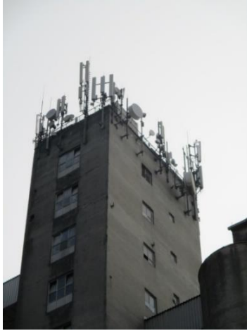
Figure 1. Collocated HF EMF sources installed on a building comprised of following systems: FM, TV, LTE 800, GSM 900, UMTS 900, LTE 1800, LTE 2100
